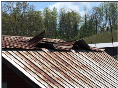
Barn roof damage from wind storm in early spring, repaired with the help of the Board of Education's Maintenance Department
